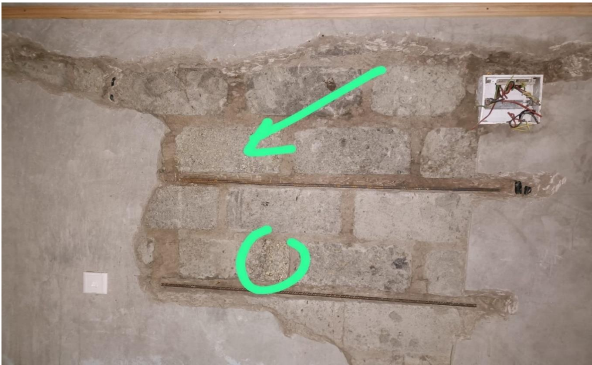
Figure 4: Noted masonry cracks on Case Study 1 (Source: Authors 2025)
