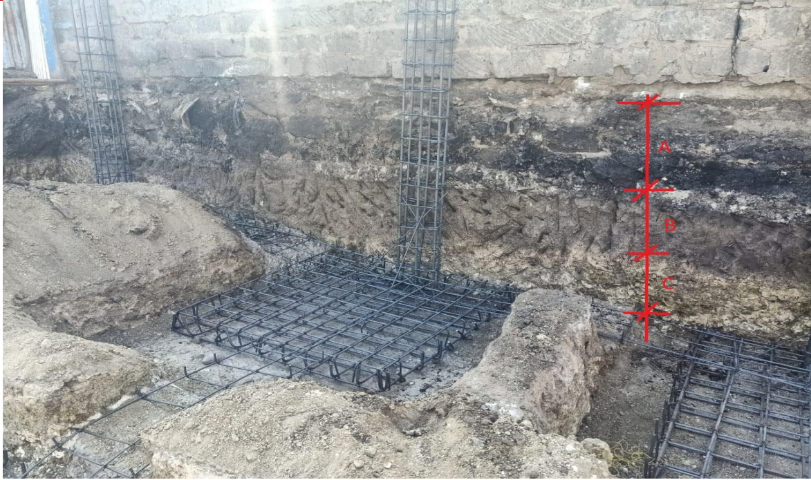
Figure 3: Differing soil strata leading to the contractor's erroneous decision (Source: Authors 2025)
